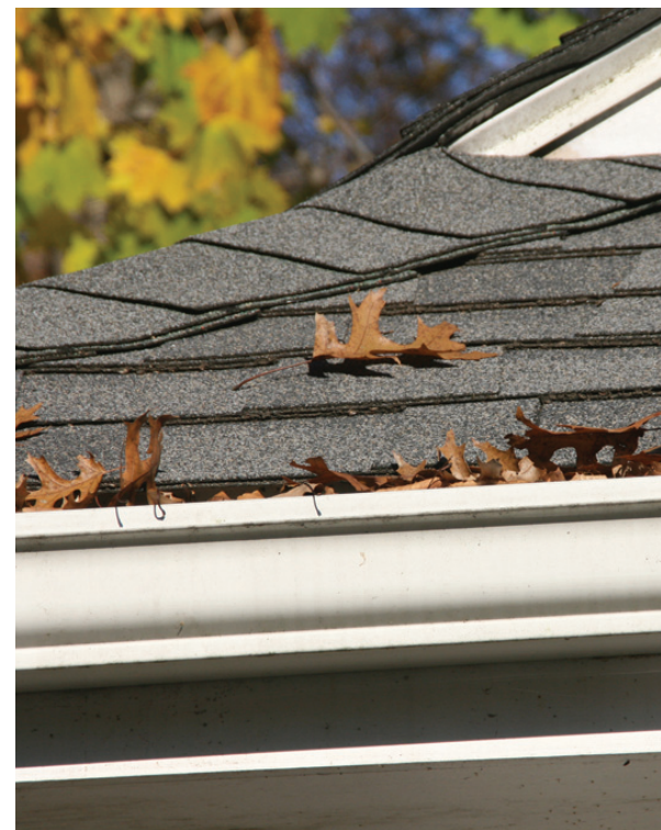
Routinely cleaning gutters throughout the fall and early winter can help reduce the risk of roof damage caused by winter weather.
